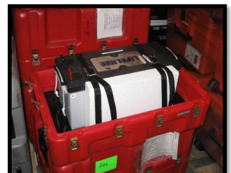
Battery strapped in place with terminal caps in a hard case.
